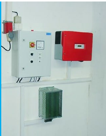
Picture 5: Upper left: control cabinet, right-side: Windy Boy from the company SMA, bottom: braking resistance
