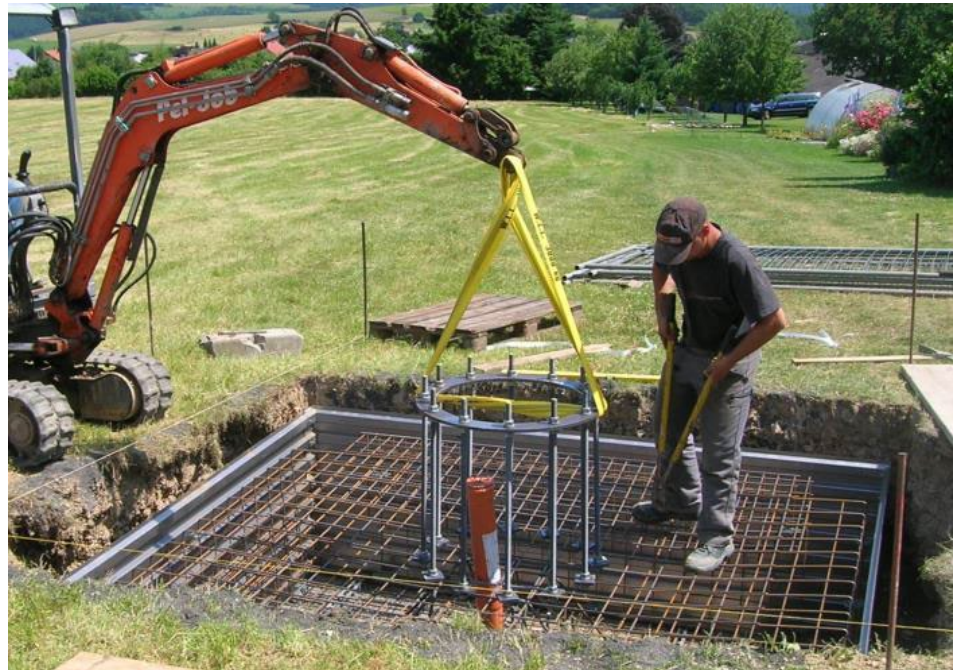
Picture 2: Installation of the lower flange (anchorage) into the fundament with the inner empty conduit for the generator connecting cable
