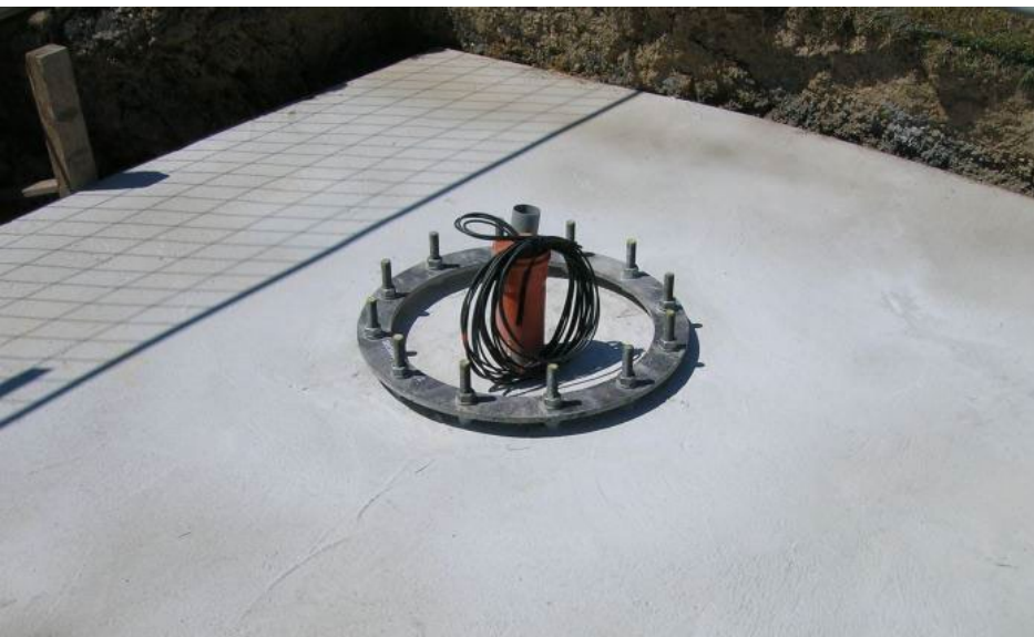
Picture 3: Ready fundament with the screws for the mast and the empty conduit for the generator connection
